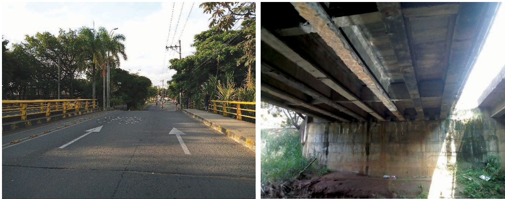
Fig. 3. Reference bridge located at 16th Street with 102-103 Avenue, Ciudad Jardín, as documented in [25].
