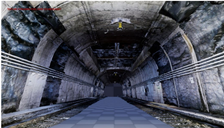
Fig. 4. General view of the tunnel in the study area in a VR environment.
